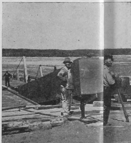
Rushing construction of new trestle to get them into service for the summer work
